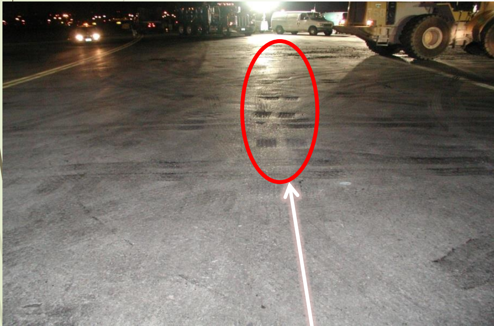
Indentations in Taxiway GG at LaGuardia Airport
